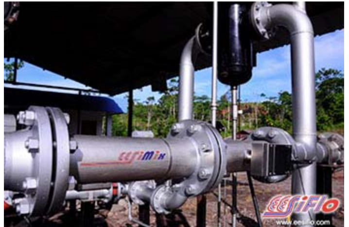
Crude Oil Export Metering Stations
