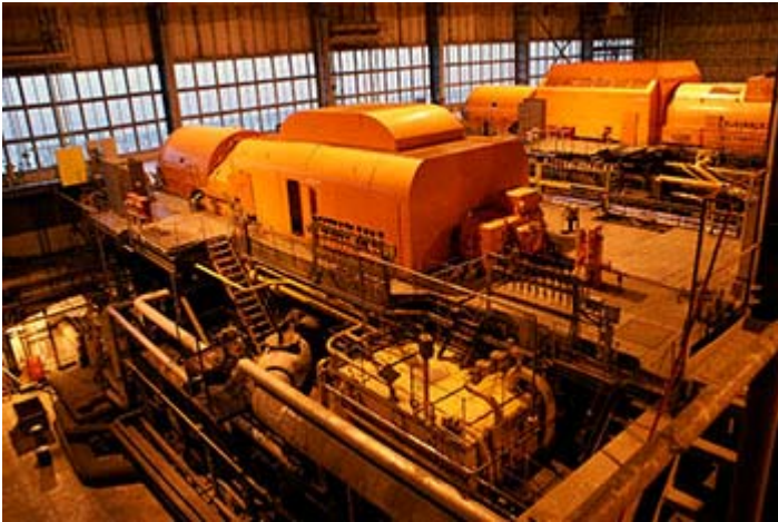
Power Plant – Power Production
